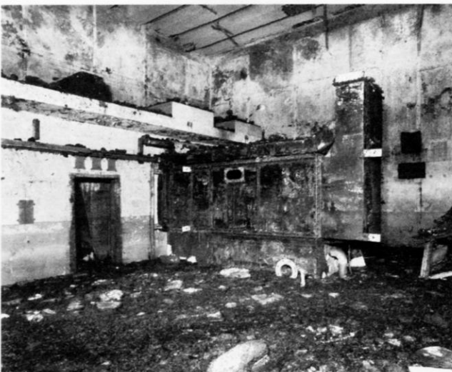
The Air Conditioning plant room. Photo by Nick Catford
